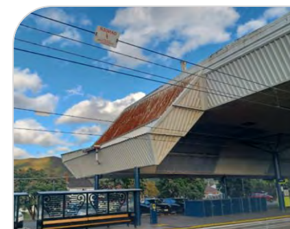
Figure 21: The lower roof pictured shows a heavy corrosion level
