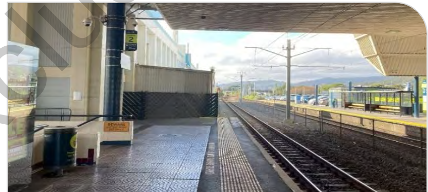
Figure 24: Tiles present slip hazard as indicated by warning signage
